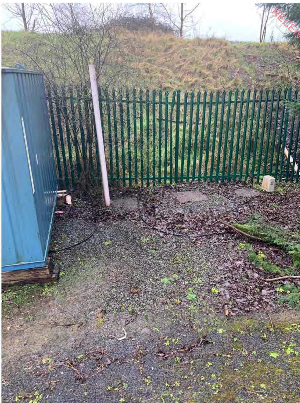
Photo 4 The Second septic tank on site serving the quarry floor's staff.
