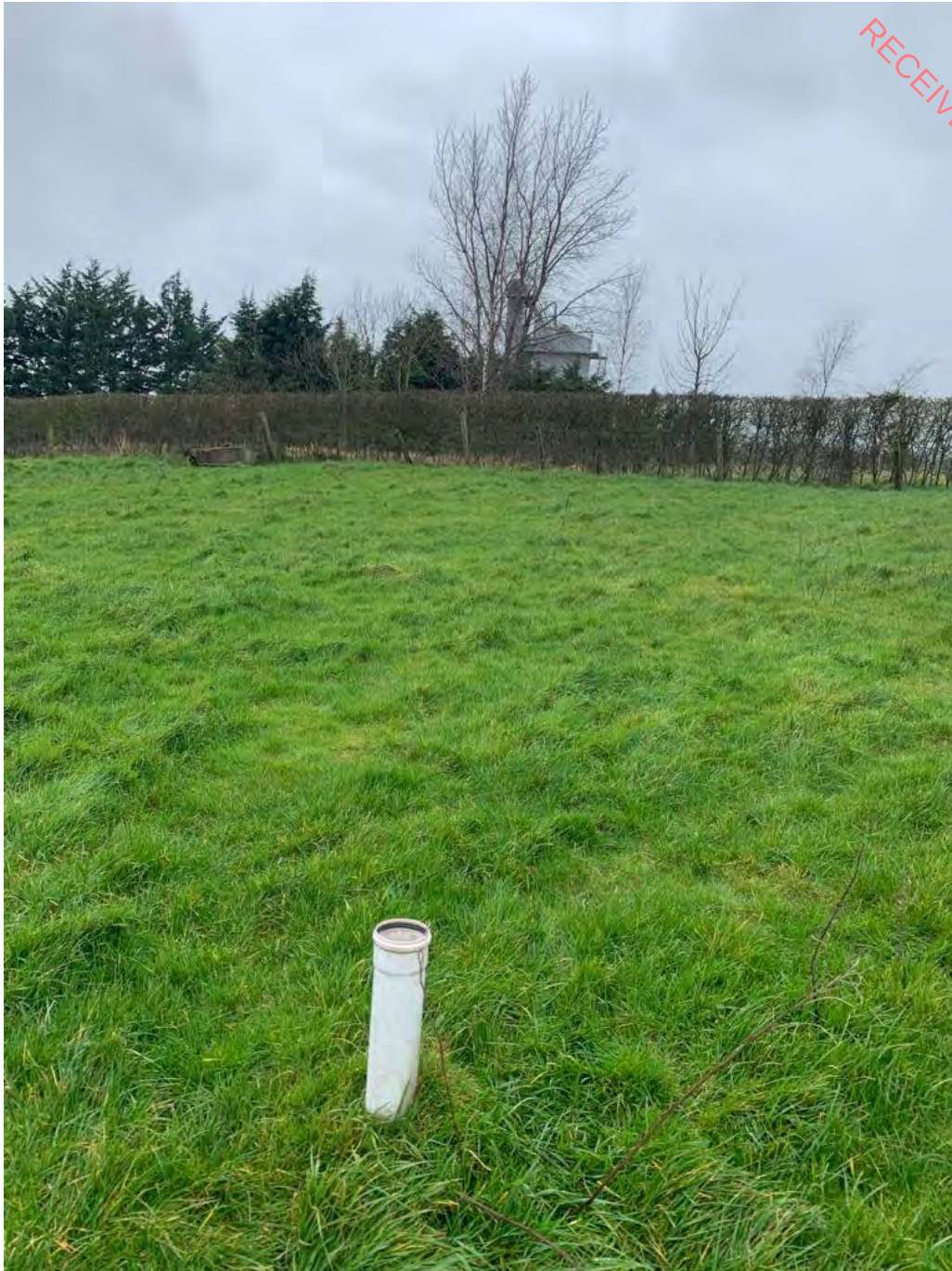
Photo 9 Vent stack for end of distribution trenches.
